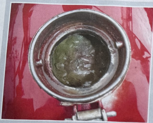
Some of the failed fuel tank liner removed
